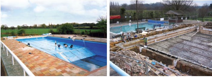
Left: volunteers cleaning the neglected site in 1984. Right: the installation of the new tank twenty years later in 2004.
